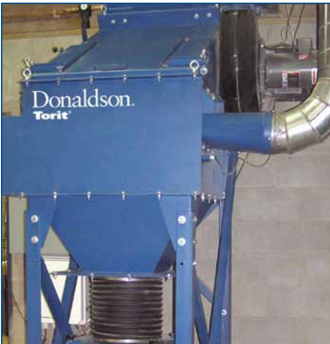
Torit PowerCore at Anchor Block.
