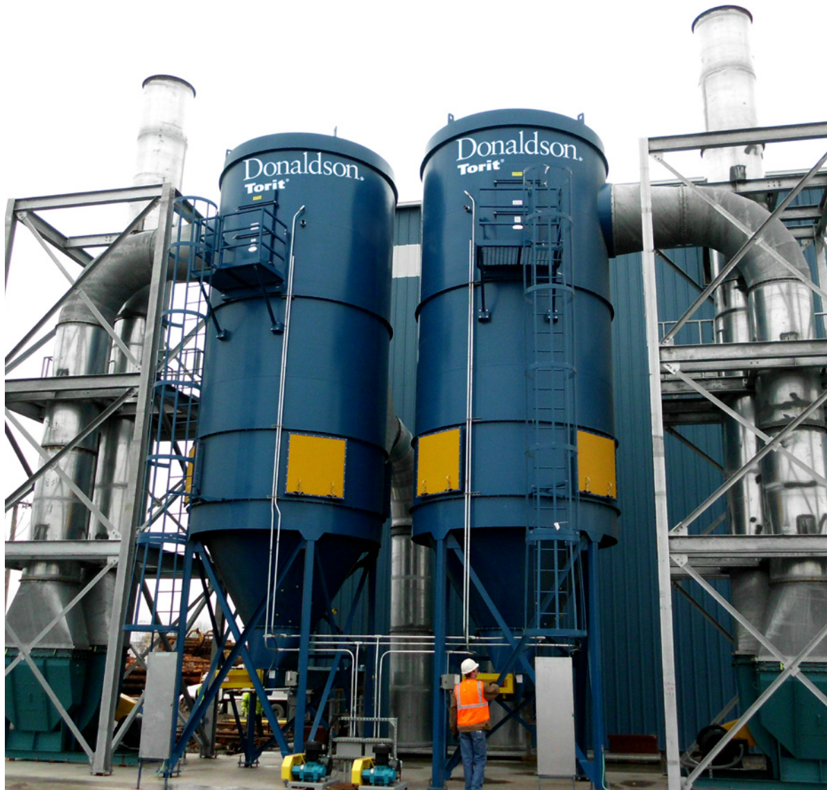
Figure 2. Traditional Centralized Baghouse Collectors
