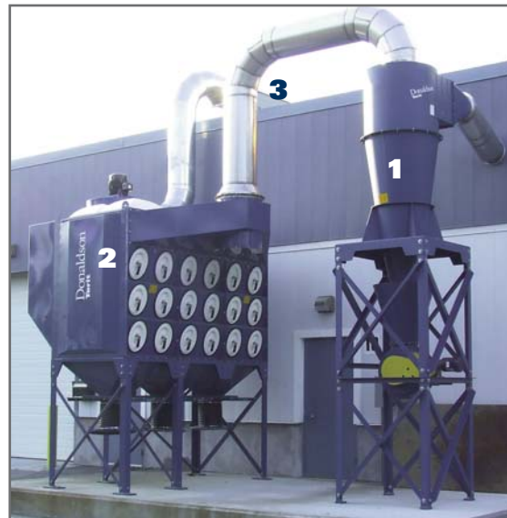
The new state-of-the-art spray booths at Falmer Thermal Spray (Salem, MA) are ducted outside the building into a (1) Donaldson® Torit® cyclone pre-cleaner, (2) then into Downflo® Oval (DFO) dust collector with Ultra-Web® filters, and (3) finally through a HEPA filter at the outlet on the roof. The system filters hexavalent chromium and other thermal spray particulate from the daily operations.
