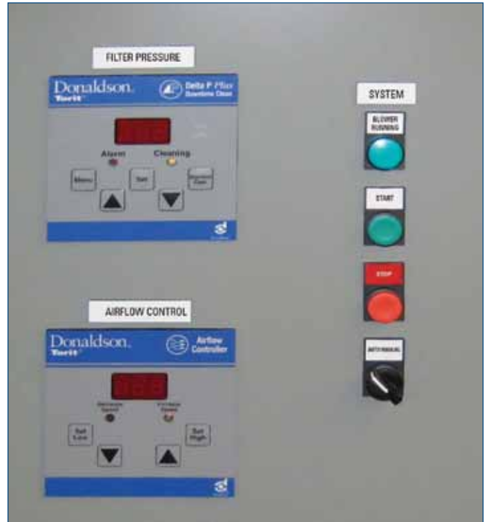
Control panel with VFD and airflow controls.
