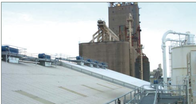
Figure 2. By distributing the dust collectors across the roof of the Southern Cement warehouse, the air in the entire building is efficiently changed every hour, which improves visibility and working conditions.
