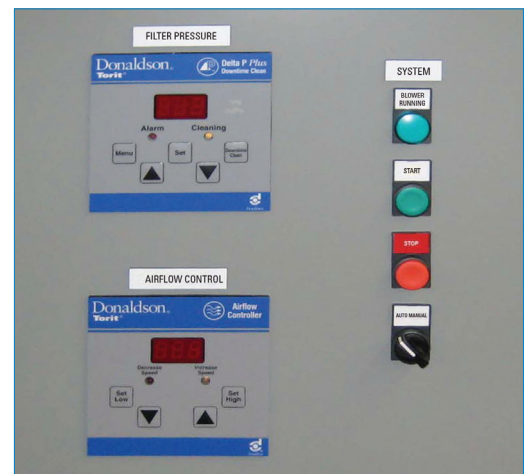
IEC Electrical Control System with Airflow Controller and VFD
