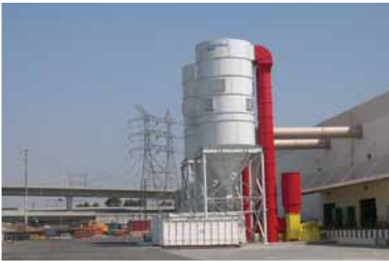
DUAL 594LP12 at door plant (180,000+ cfm/combined)
