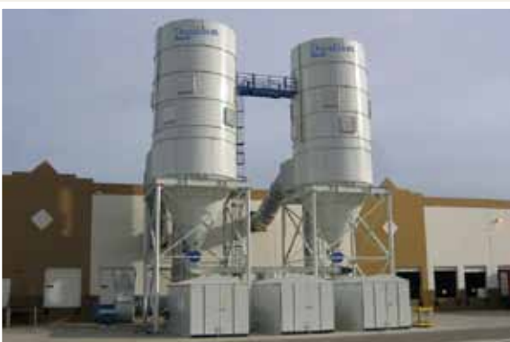
Two 594LP12 at a cabinet plant (80,000 cfm/each)
