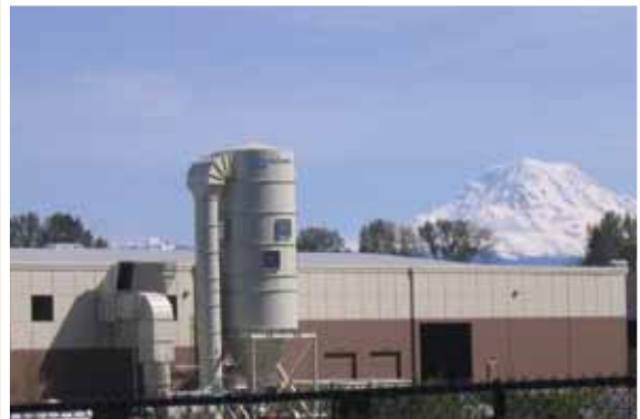
528LP12 at cabinet factory (70,000 cfm)
