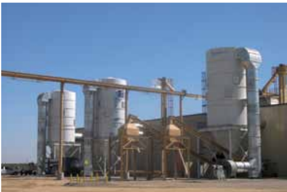
THREE 684LP12 at almond shelling plant (100,000 cfm/each)
