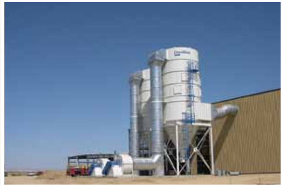
882LP12 at almond plant (140,000 cfm/each)
